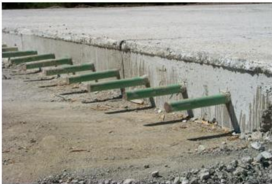
Figure Dowel bars in place at a construction joint- the green color is from the epoxy coating.
